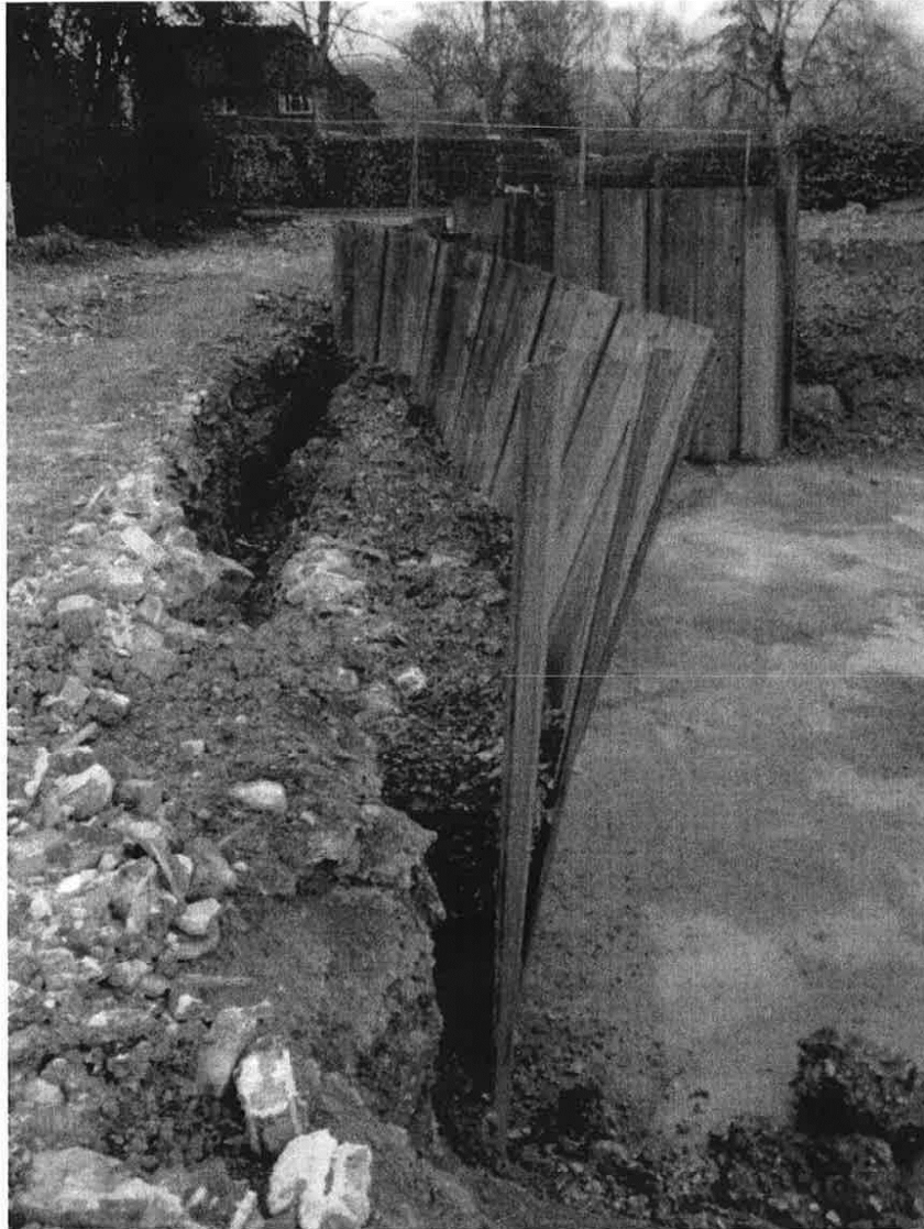
This picture is of the ground to the Western boundary, but the same thing happened to the eastern boundary piling, though for some reason I don't have a picture for this.
